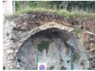
Photo 2: Ravello: A collapsed vault
